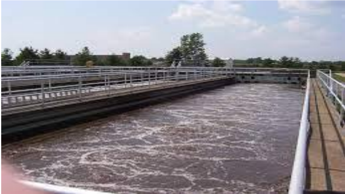
figure (4) wastewater treatment basins
